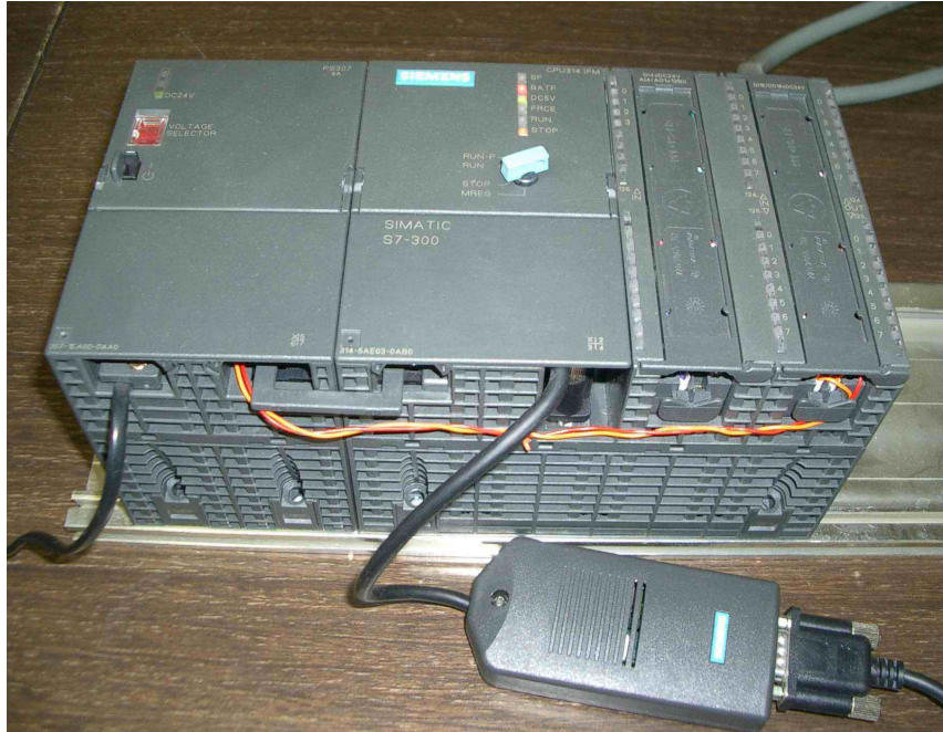
Figure 7.2: Laboratory control system with PLC CPU 314 and power supply
