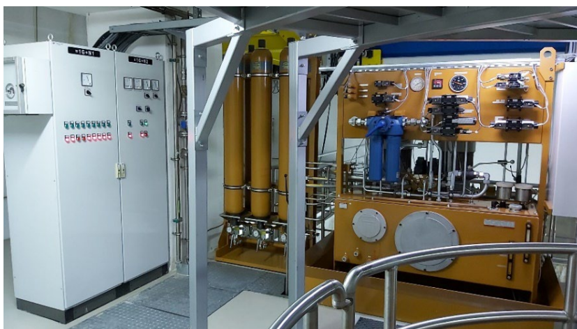
Figure 5: Hydraulic power unit.
