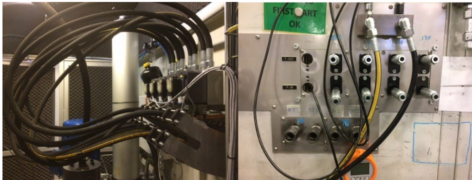
Figure 4: Additional flow meters which are easily to grab and plug into the tested valve.
