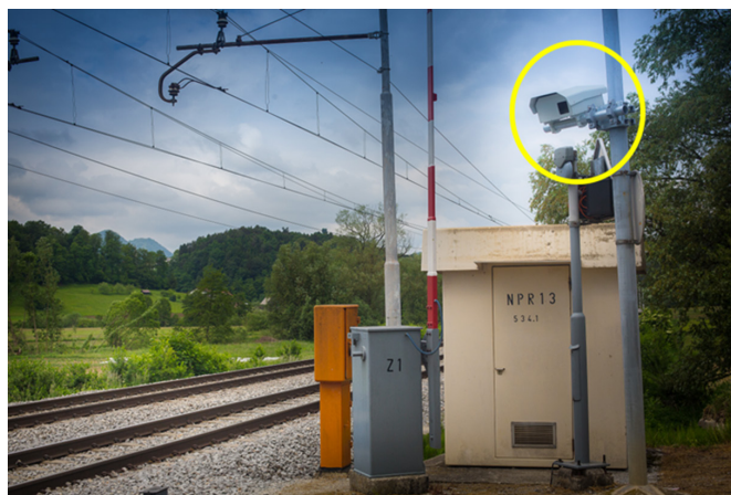
Figure 30: LiDAR sensor (in a yellow circle) installed on a pole at the level crossing (Foto: archive of FOKUS TECH d.o.o.).
