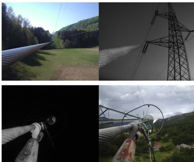
Figure 3: Camera installed in OTLM device; Source: (Gubelj, Lovrenčić, Bakič, et al., 2020)
