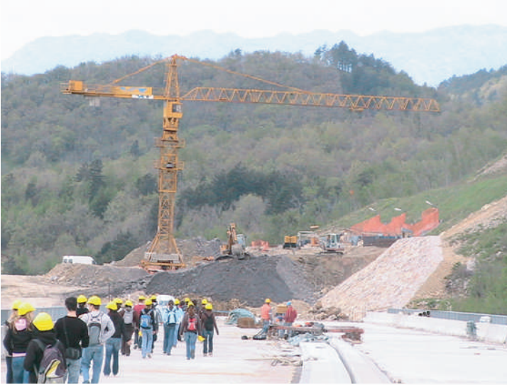
Excavation of three caissons in order to improve security conditions in a deep excavation cutting between profiles P284 and P294 at the highway section Razdrto - Vipava
